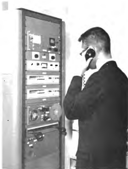
FIG. 19. Spot news recording center, which permits recording off telephones, 2-way radio, or from News Booth control. Equipment includes RT-7 Cartridge Tape machines and NBC Hot-Line alert receiver.
