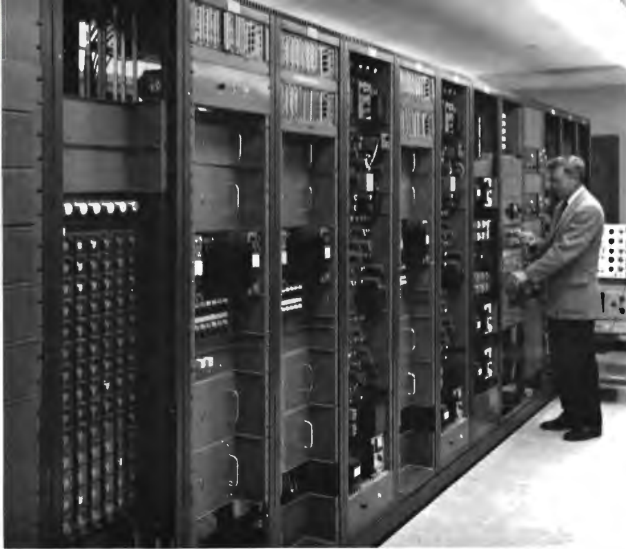
FIG. 31. Rack equipment in control room includes BA-33 Transistorized Audio System and three TS-40 Transistorized Switching Systems. (Provision has been made in switchers to accommodate 4 live color cameras, color film chain, and another TR-22.)
