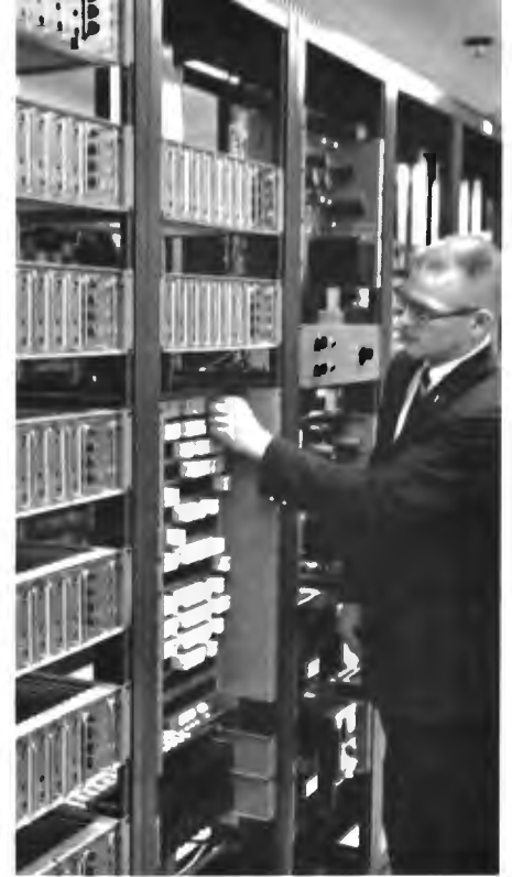
FIG. 32. WOC-built house monitoring system distributes 15 video sources to 15 offices and special areas. At left, are new RCA TA-24 Transistorized DA's (Pulse and video distribution system are completely solid-state.)
