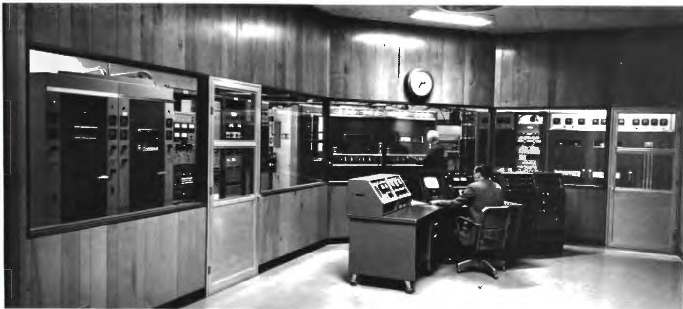
▲ FIG. 36. AM and FM Radio and TV transmitter installation. Radiating 100 KW on Channel 6, WOC produces highest signal strength in the area.
